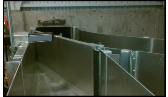
Exlar's Tritex II actuator installed on one of Portland General Electric's fish diverter doors.
